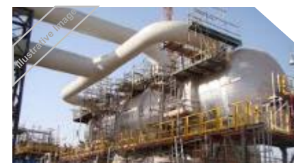
MEP for Bu Hasa Oil Project (Tecnicas Reunidas) AED 521 million
